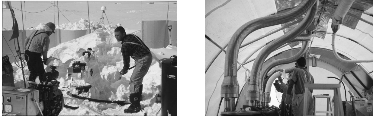
Figure 2. Plant and equipment digout during drill trial season (left), exhaust ducting from 80 kW heaters inside new plant shelter in current set-up (right).
